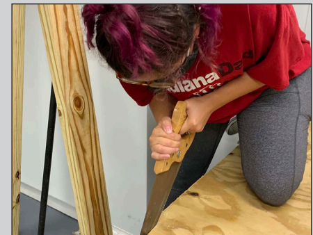
Victoria Lydick trims a plywood shelf with a handsaw during the construction of the facility. Photo courtesy of Julia van Kessel
